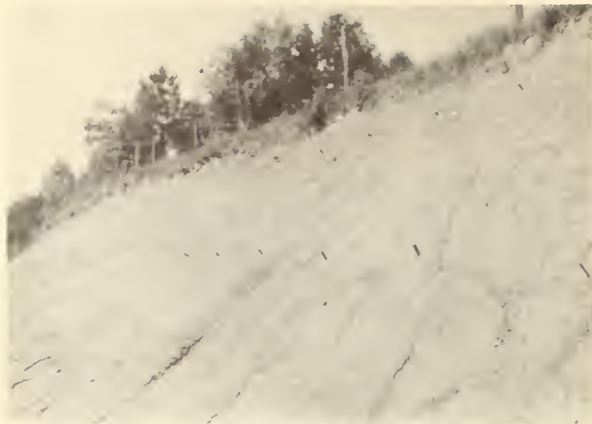
Figure 10.--A part of the two rows of metal pins driven into the bare bank until the tops were flush with the soil surface when the plots were established. After 2 years of erosion the pin tops are from 0.02 to 0.35 foot above the soil surface. The soil loosened by frost action has been washed from the upper part of the bank leaving it relatively firm.
